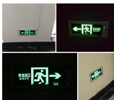
Figure 1. Traditional emergency evacuation light.
