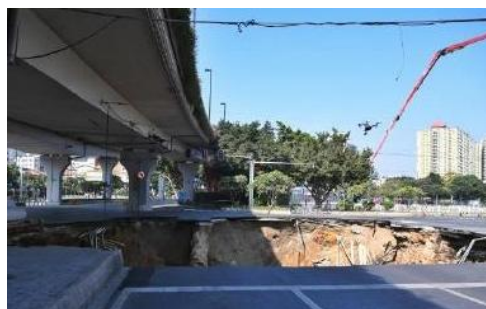
Figure 2. Collapse Accident of Deep Foundation Pit.
