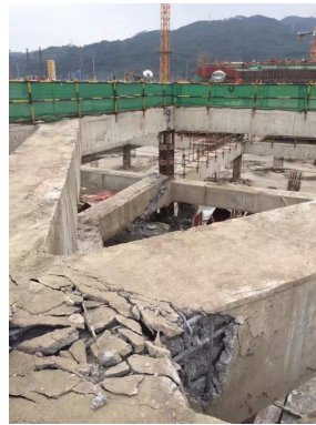
Figure 1. Example of a “Kicking” Accident Caused by Mud Sliding in Deep Excavation Works.
